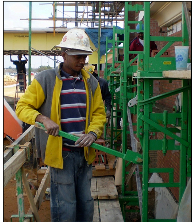
The Jack Handle moves from tower to tower and jacks up the masons and their workbench together.
