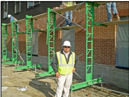
"We can move 105 feet of Workhorse to the next wall in 20 minutes." Carlos Reyes, WT Construction, New Orleans, LA
